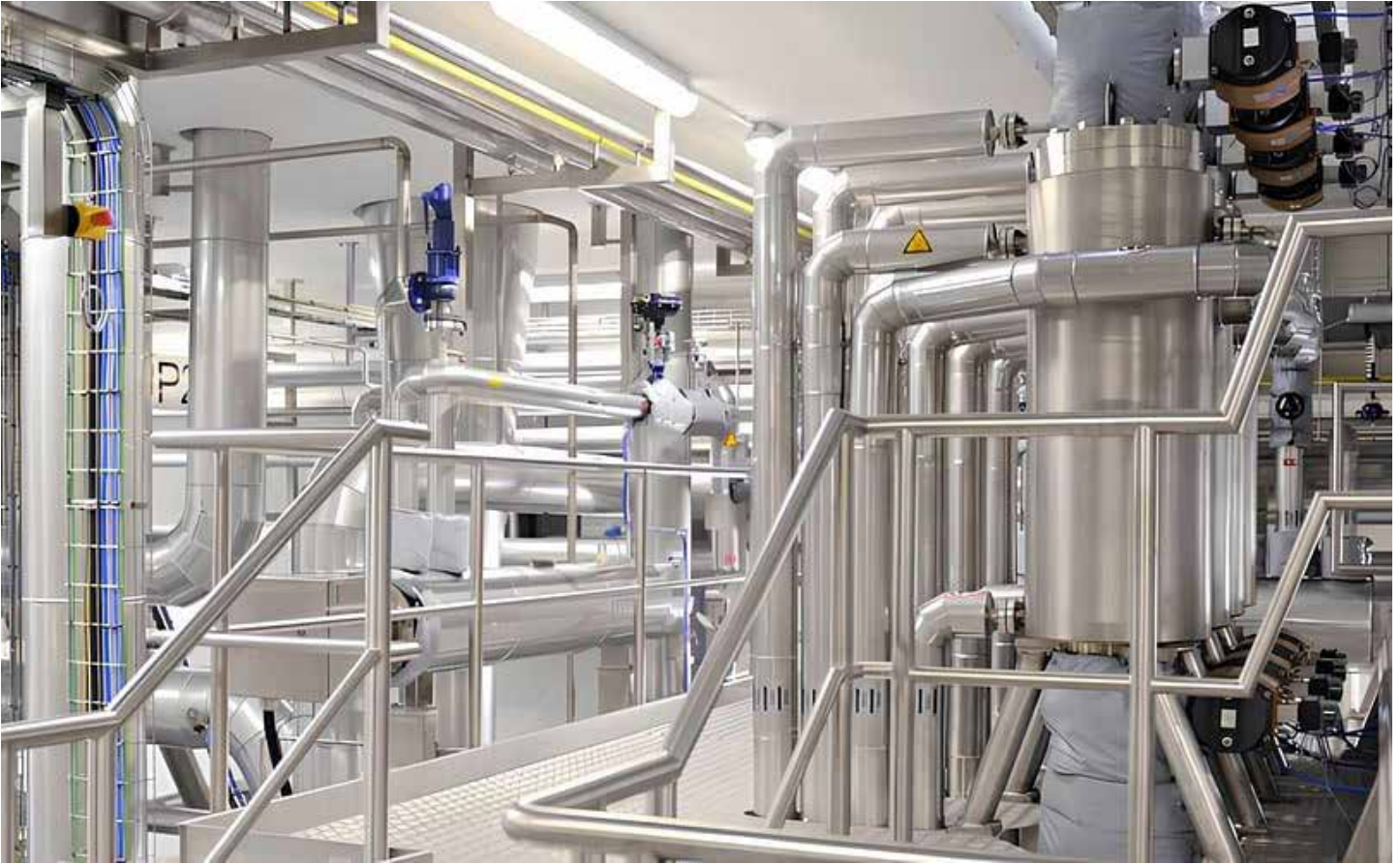
Puffing system reactors: it eliminates the disruptive "gunshot noise" typical of older systems.
