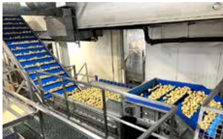
A closer look at the advanced potato processing system at Burgess Farms, featuring Haith's innovative washing, drying, and sorting equipment, designed to optimize quality and sustainability.
